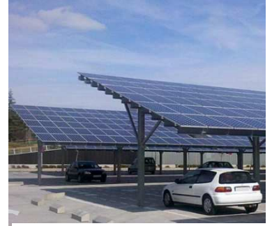
Figure 3 : Ombrière de parking (source : wikipedia)
